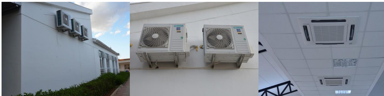
Figure I.2.3.25 Newly renovated cooling and heating system in the E 1 and 2 block studios
